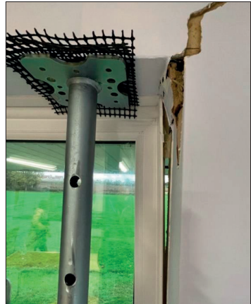
Supports in place propping up the roof. Daylight can be seen between the window frame and the wall which indicates the extent of the subsidence...
